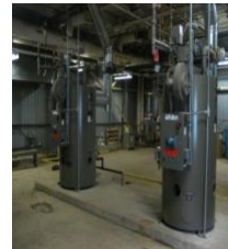
High Efficient Boilers Picatinny Arsenal, NJ
