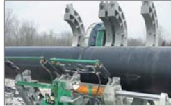
Geothermal Cooling System Engine Manufacturing Client, Lima, OH
