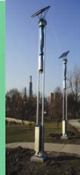
Wind and solar powered pedestrian lighting in a Chicago park
