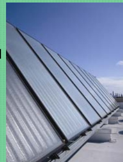
Solar thermal panels atop the Rosa Parks Apartments
